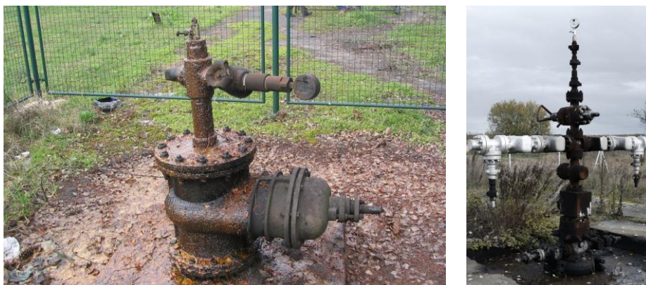
Picture1.25 Examples of the appearance of above-ground equipment of geothermal wells (Gaurina, 2022)
